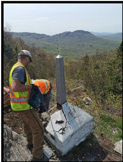
Figure 9: Karl Leblanc prepares Monument 592 for repairs, located at the end of the Long Trail. (QC/NY)
