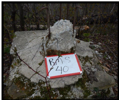
Figure 4: Reference Monument RMS-40 found deteriorating in the forest along the shore. (NB/ME)
